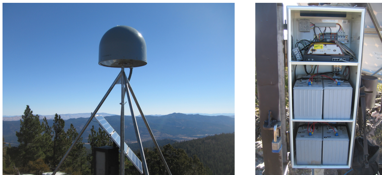
Figure 7.3: Example of PBO hardware at p147 in northeastern California. The stations are equipped with a Trimble NETRS receiver and a choke-ring antenna.
